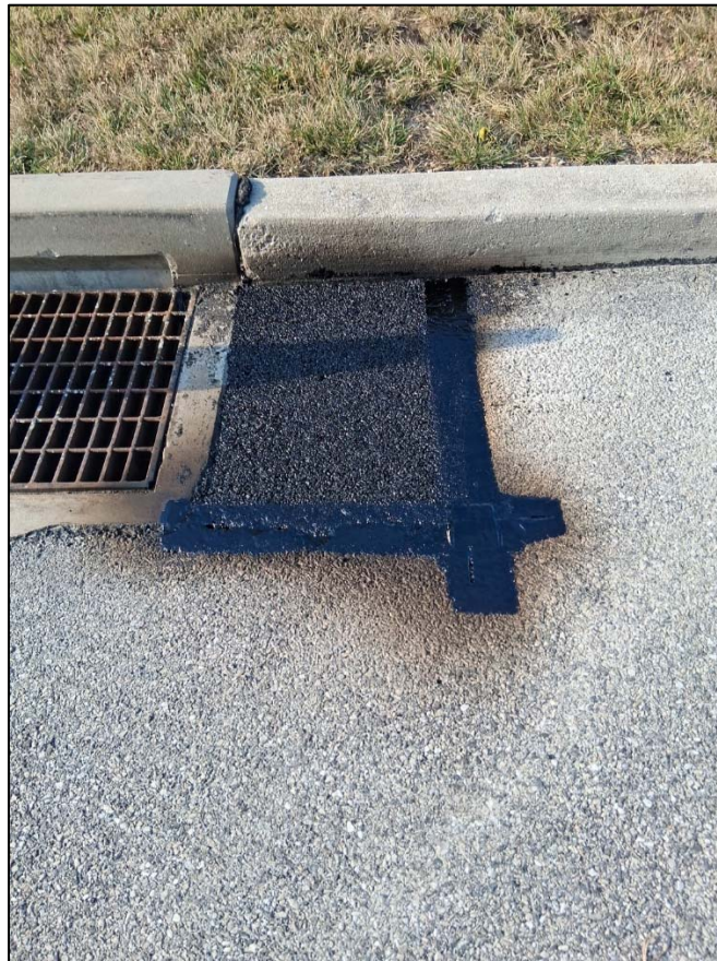
Photo of asphalt cap with seams filled.
