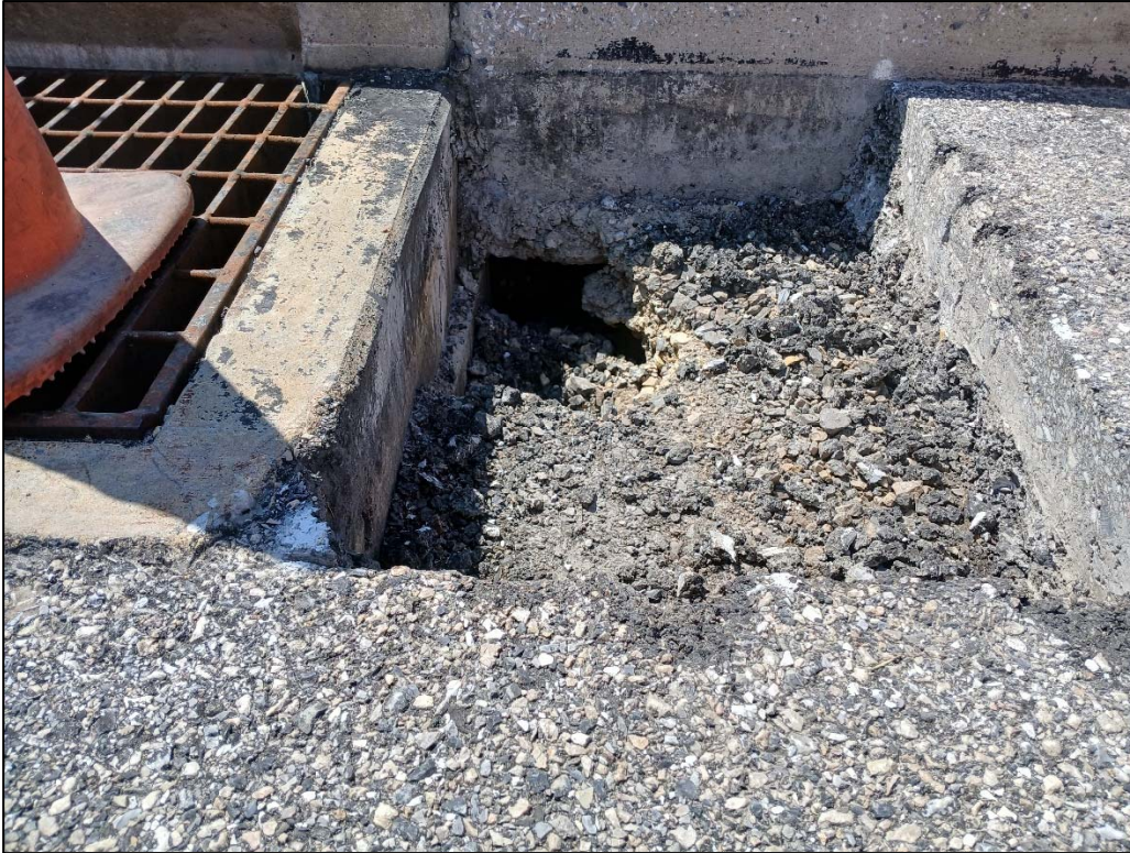
Photo after the asphalt around the sinkhole was removed.
