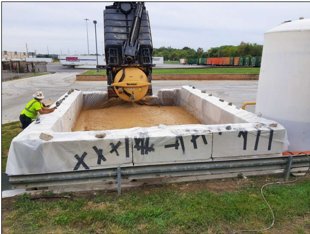
Hydrovac material dumped in salt storage area.
