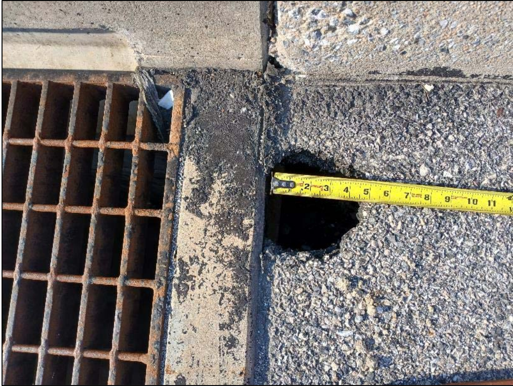
Photo of the sinkhole adjacent to the stormwater inlet.
